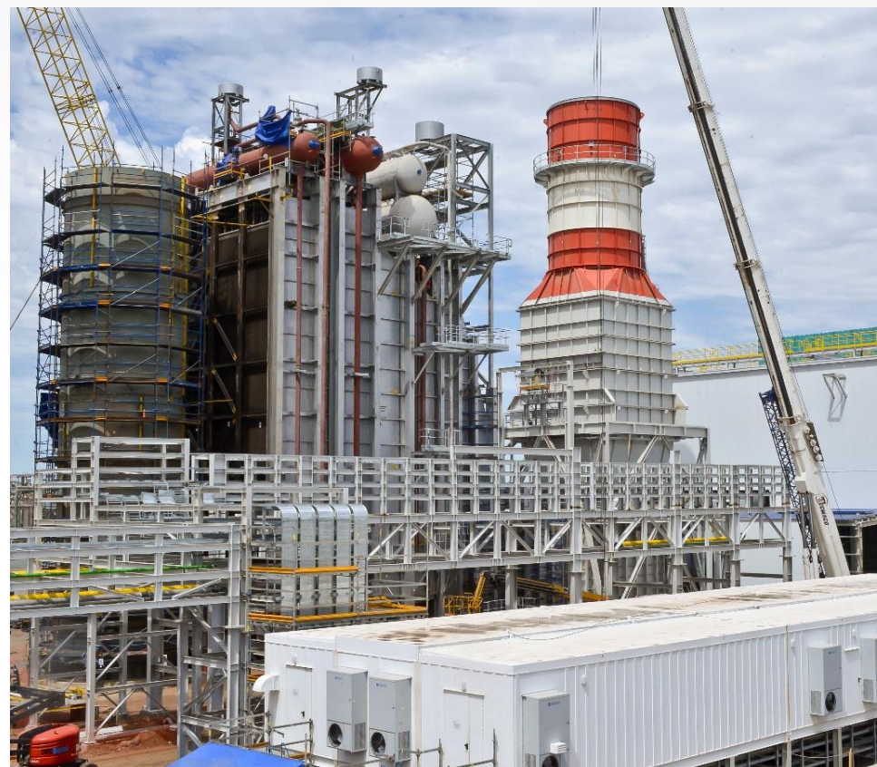
Uses 1 of the 4 turbines already purchased by Central Puerto
